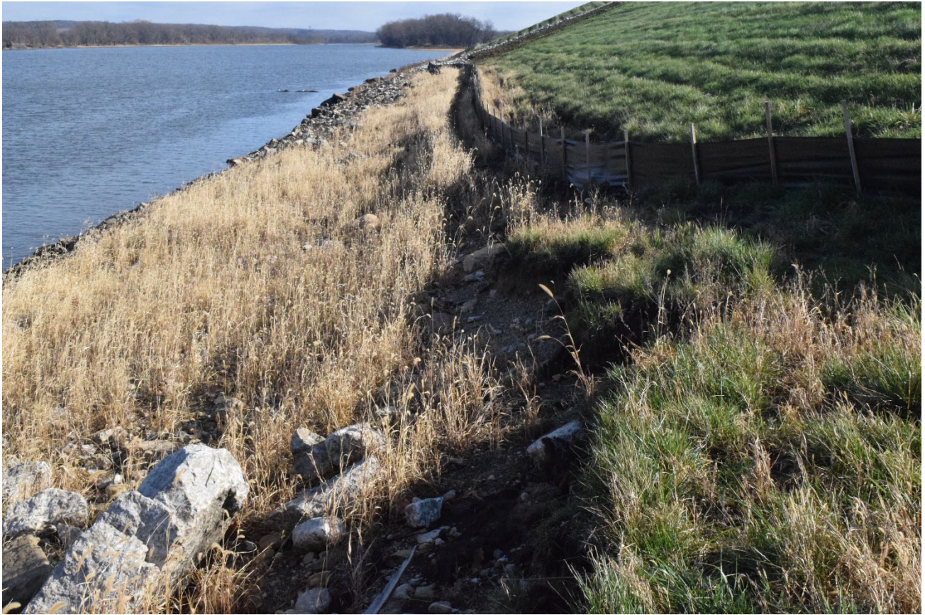
North side adjacent to river – repair erosion
