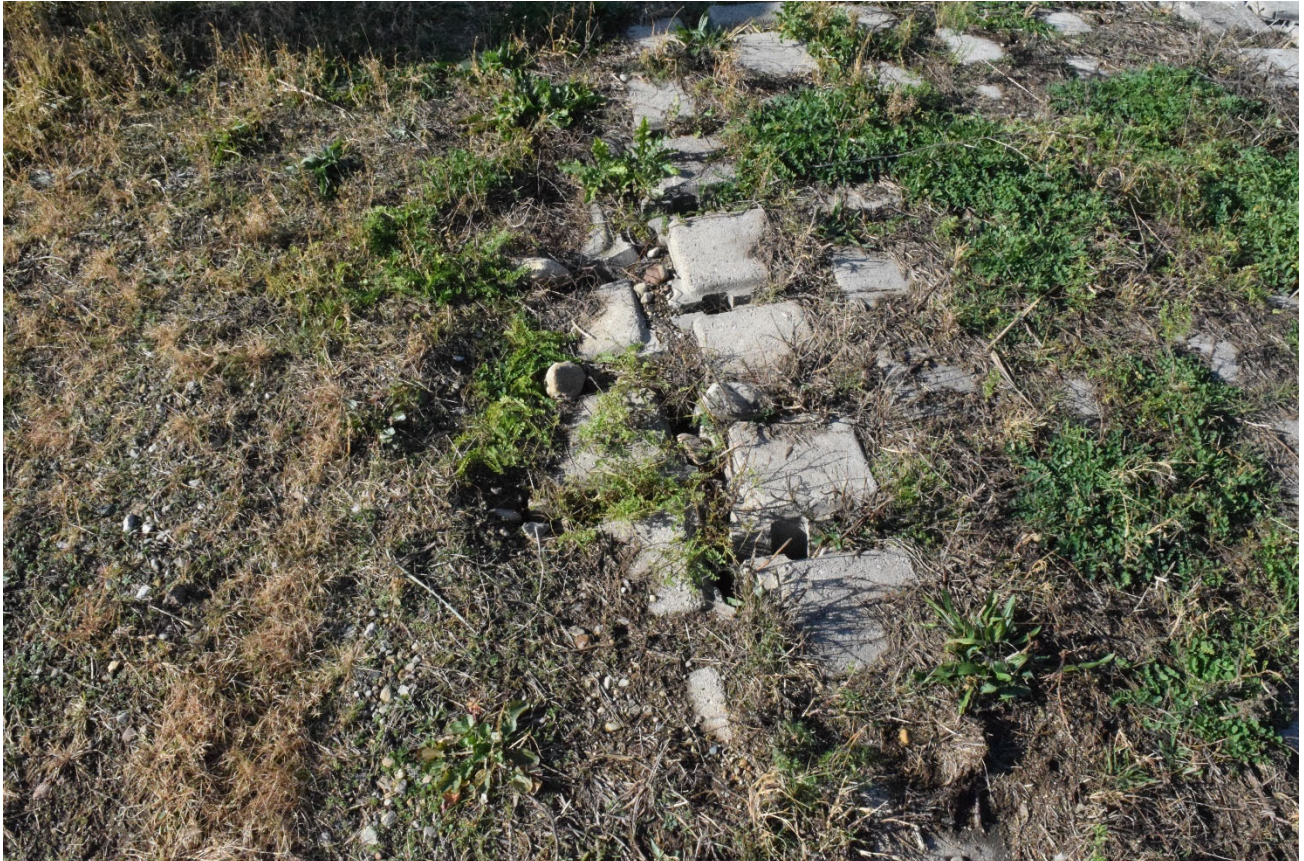
South side new pond – aggregate missing – fill voids between blocks
